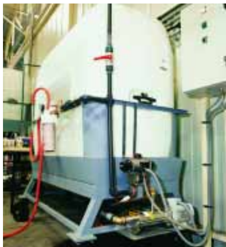
Compact M2200C4 for feeding salted water installation.
